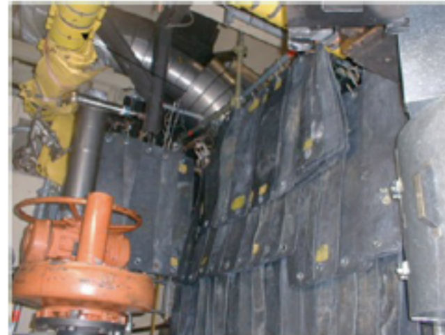
“Bracelet” type protection on a pipe
