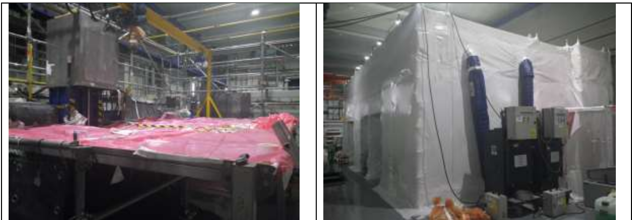
Figure 3: Left: table for the waste treatment. Right: confinement made of a scaffolding covered by a thermo-retracted skin
