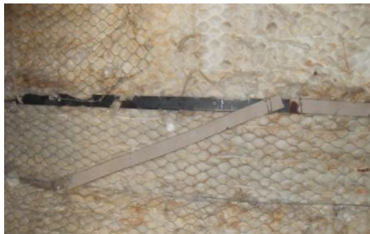
Figure 7 - Condition of the asbestos fibres in the insulation of the old steam generators.
