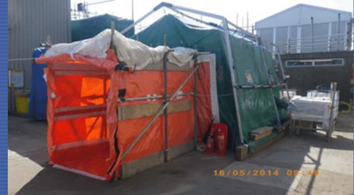
Bradwell (UK): example of a typical temporary structure used for a contamination area work
