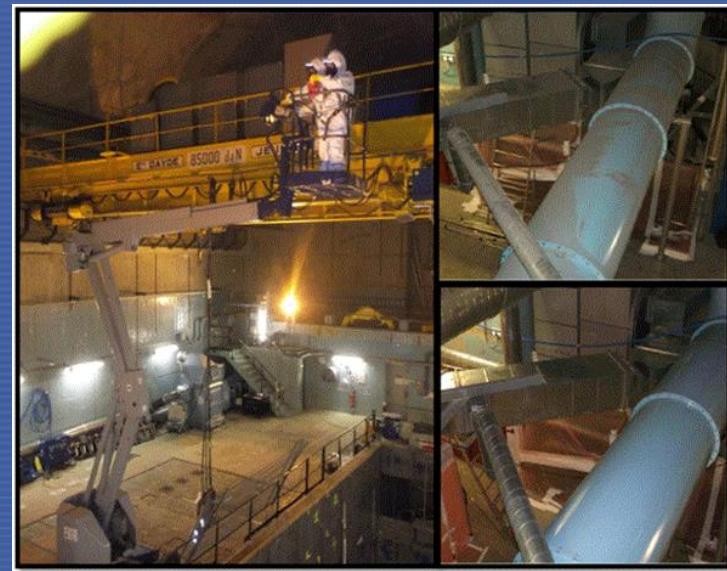
Chooz A decontamination (2014) Left - decommissioning of the fuel building Right - pipework before and after cleaning
